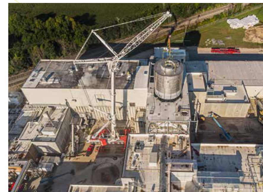
The Liebherr LTM 1500-8.1 and the versatility of its VarioBase® outriggers move in close in tight quarters to set a 121,000-pound dryer at a dairy production line in Wisconsin.
