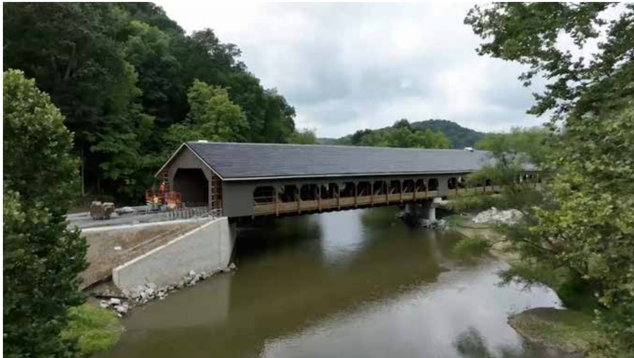
This latest Video Case Study demonstrates how ALL used two all-terrain cranes – a 770-ton Liebherr LTM 1650-8.1 and a 550-ton Liebherr LTM 1450-8.1 – to help customer Kokosing Construction build the new bridge in the middle of one of Ohio’s largest camping and recreational centers.
